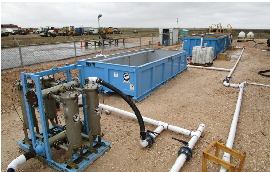
A nanobubble-based wastewater treatment system operating for Permian Disposal Services in Texas. The system’s developer says it is treating about 11,000 B/D day of produced water and enabling the operator to recover nearly all of the 2-3% of oil (by volume) that is mixed in with the water. Photo courtesy of Nano Gas Technologies.
